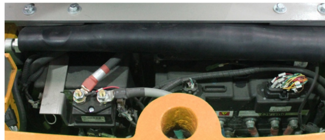
Open the balance heavy cover, you can control the electrical maintenance.
